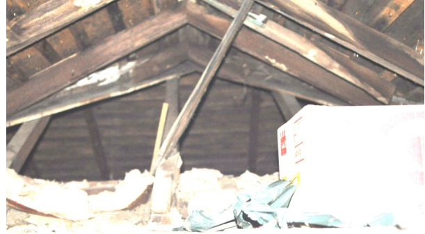
Attic view photo showing rafters taken from an access door in the east bedroom ceiling looking west.
