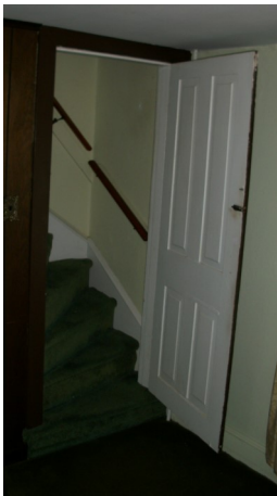
View of the base of the winder stair leading from the living room to the upstairs bedrooms.
